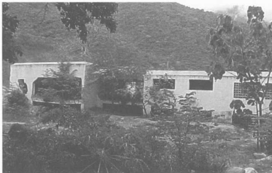
Bolivarian School after the 1999 torrential flow
