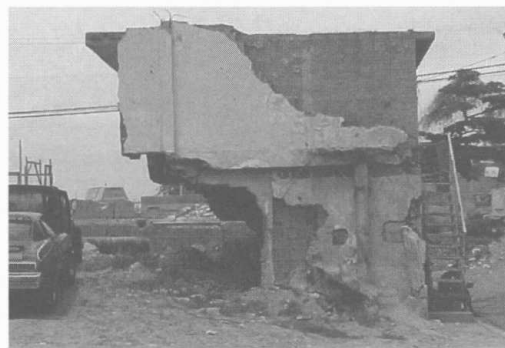
House affected by the 1999 torrential flow
