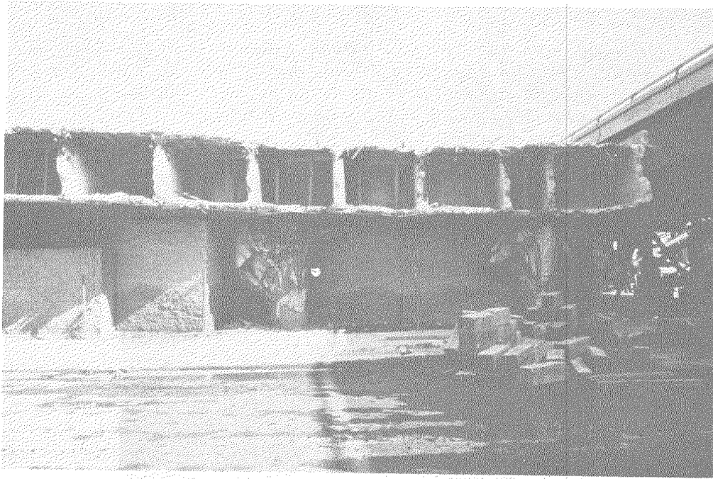
Fig. 29 Impressive buckling of steel bars and concrete crushing along the height.
