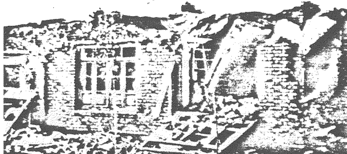
Collapse of dispensary due to earthquake of September, 1st, 1962 in Buin-Zahra (Iran)
