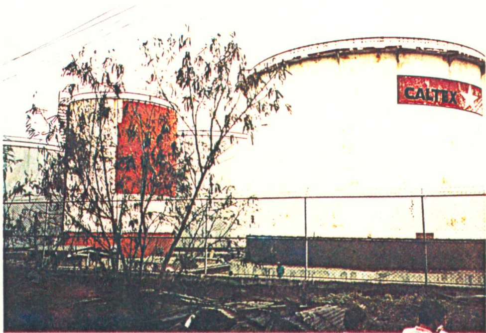
Photo 4.30 Damaged oil tanks in the port of San Fernando. Red portions of the tanks at the lower part (left and right tank), and the upper part - right side tank are indicating damaged parts.
