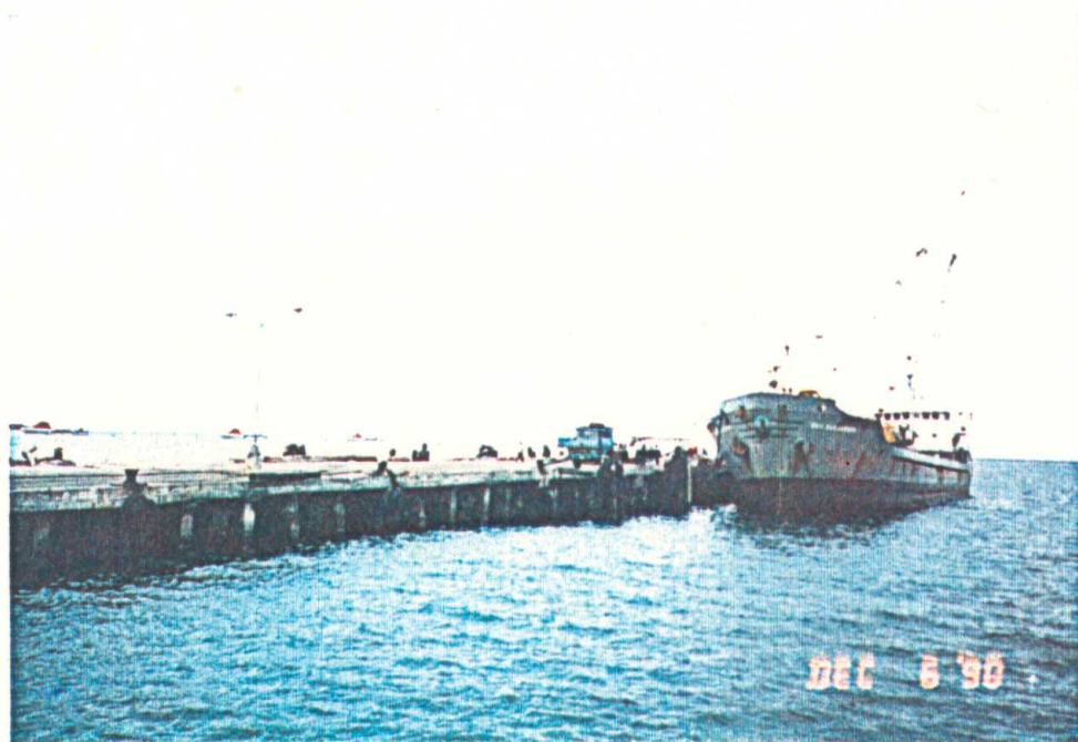
Photo 4.28 Side view on pier No. 1, port of San Fernando. Tilted substructure of the pier by more than 7 degrees toward the sea. Plastic hinges observed at the top of the piles indicating failure in the flexural mode.
