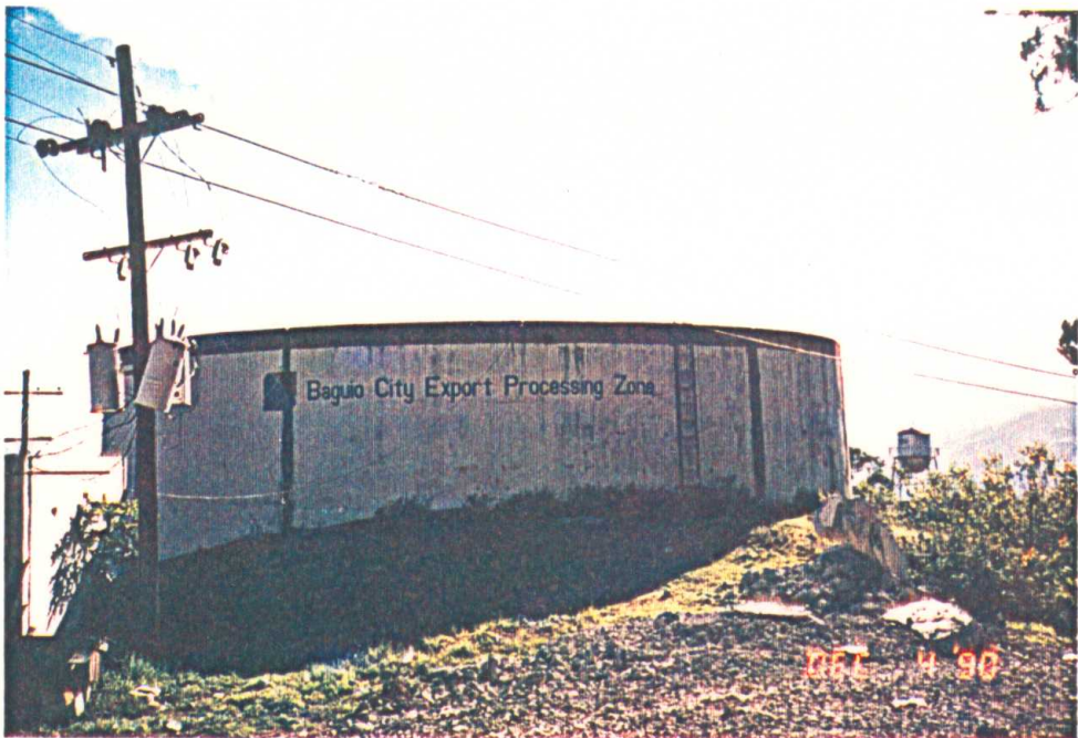
Photo 4.26 Reinforced concrete tank in the Export Processing Zone of Baguio City. No damage is observed, reported failure and heavy damage of the production and storage buildings in the same zone.
