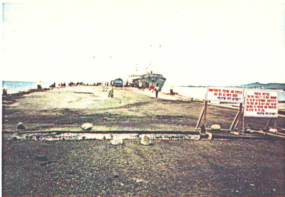
Photo 4.27 Extensive damage in the pier No. 1 in the port of San Fernando. Separation of the pier deck from the shore by 80 cm; intensive settlement and tilting towards the sea.
