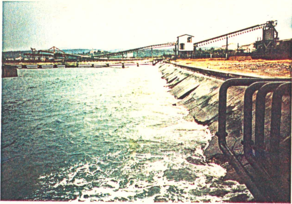
Photo 4.29 Damaged embankment cover at the shore, port of San Fernando.
