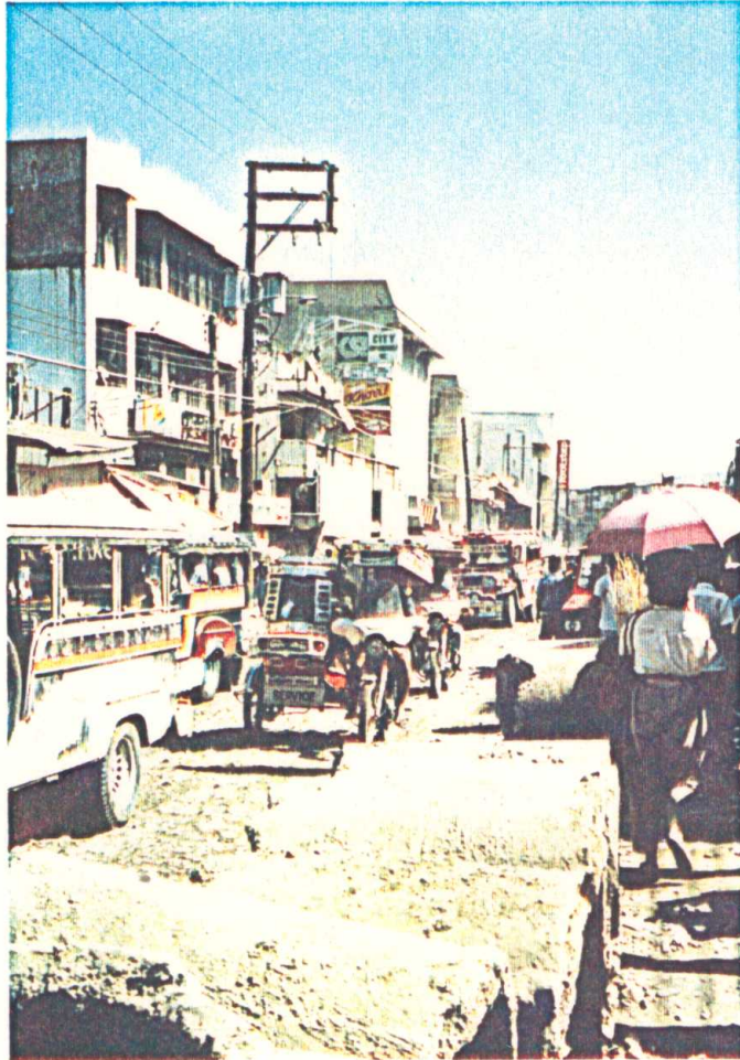
Photo 4.23 View on the Hernandez Avenue and concrete pipes taken out from the sewage line in Dagupan City.
