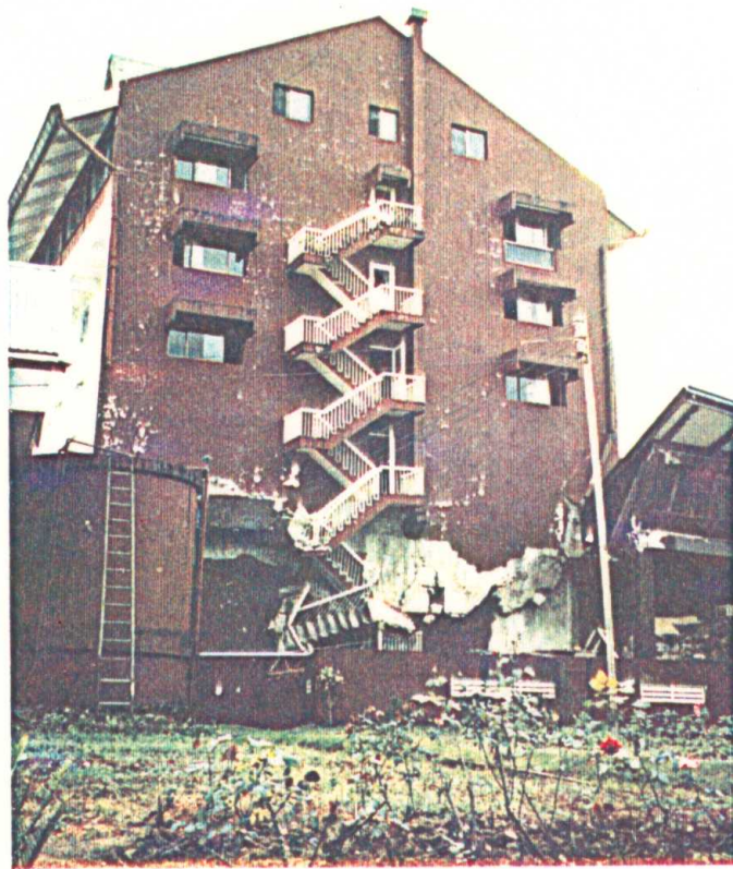
Photo 4.12 Failure of six story Country Club (Baguio City) second floor completely collapsed due to failure of r.c. low ductility frame, deep lintel beams and pronounced torsional effect.
