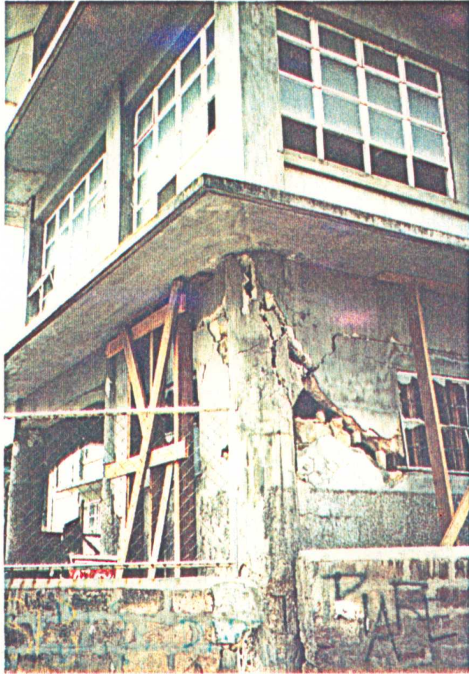
Photo 4.15 Shear mode of failure of r.c. column in the ground floor of the 3-story school building shown in the previous photo.
