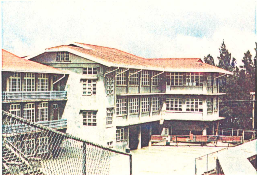
Photo 4.14 Partial structural damage of a 3-story r.c. frame building sited on a low inclined slope (St. Louis Girls High School, Baguio City).
