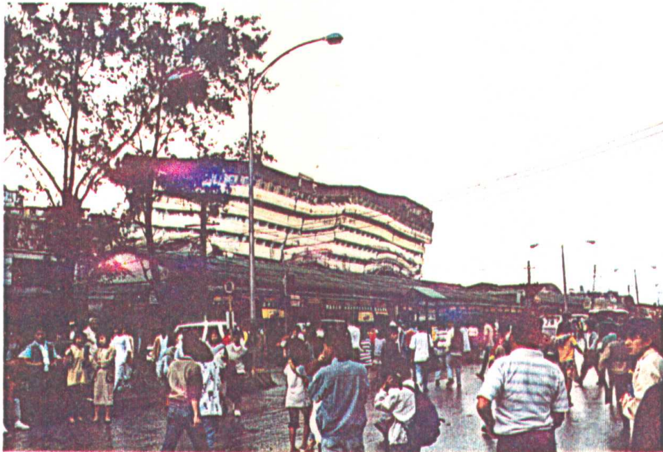
Photo 3.2 Collapsed Hilltop hotel, 7-storey r.c. building, in pancake mode of failure due to nonductile r.c. frame structure, heavy floor structures and deep facade (lintle) beams.
