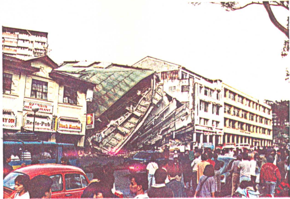
Photo 3.3 Collapsed Park hotel, 7-storey r.c. building, between effectively undamaged buildings on the same street. Typical brittle failure of load carrying structural system and heavy floor structure.
